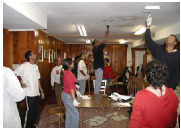
Final touches to the basement ceiling after a day-long effort by eager volunteers.
